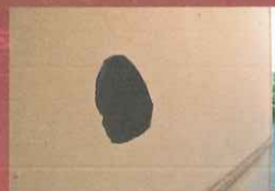
Holes in fibro walls
