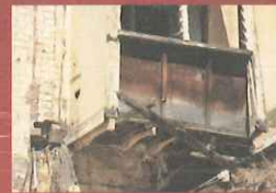
Exposed asbestos after a fire
