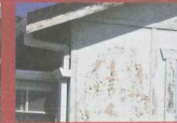
Exposed asbestos due to peeling paint
