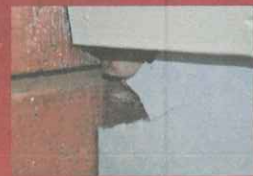
Damaged Tilux in bathrooms or laundries
